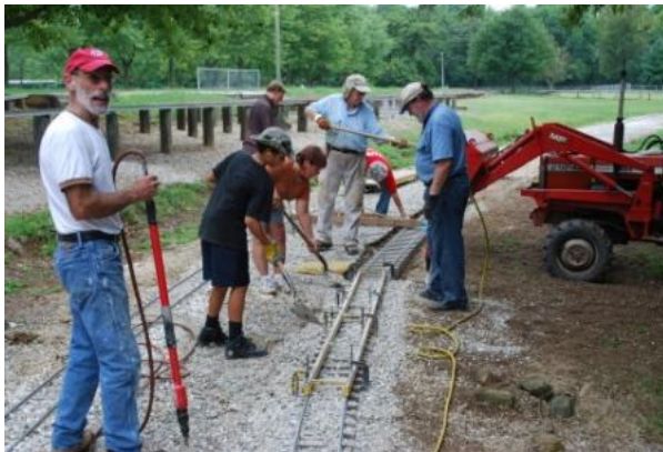
Another at Brace Junction
