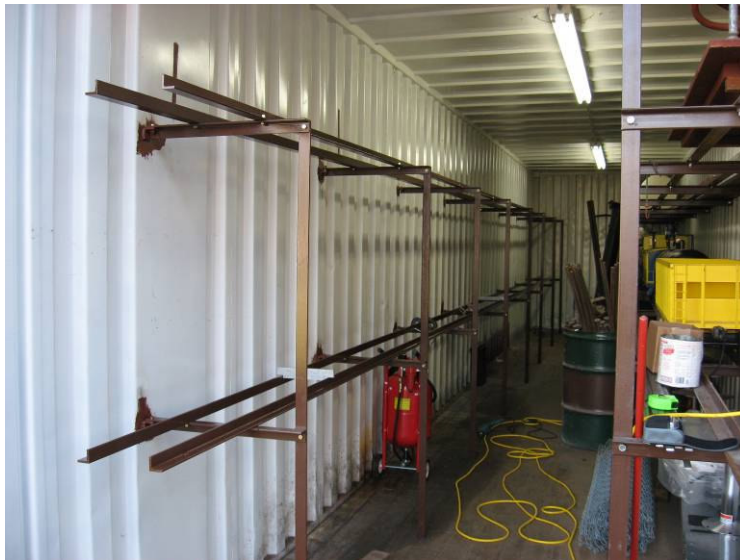
Bob Schwoerer Has Been Busy Building Rack #2 in Container #2 for Car Storage
