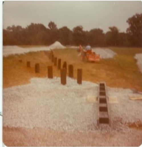
Left: Working on lead from yard to lift. Air compressor used before Midway was built.
