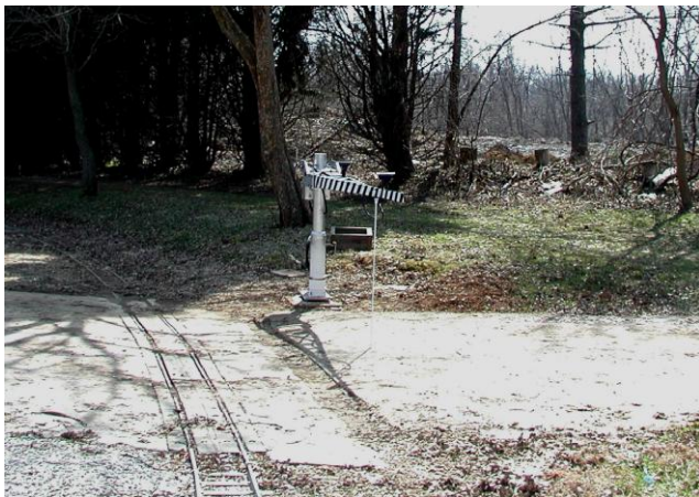
(3) Condition of the Outside Track Is Poor
