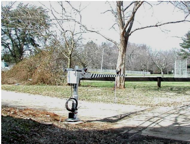
(1) Working Parts Are Missing or Hanging Out
